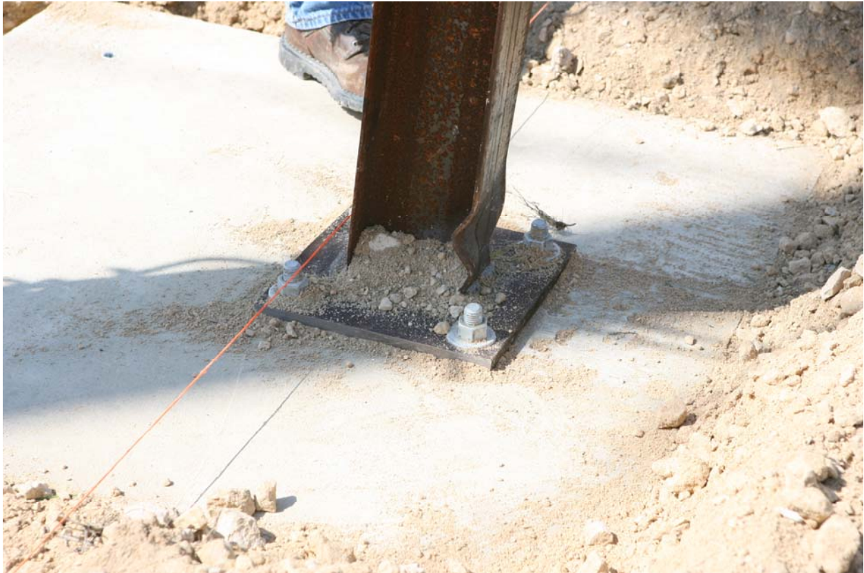
Figure D4. Steel posts over underground structure with 48-inch concrete footing after test 405160-12 P2.
