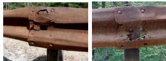
Visible Signs of Corrosion
