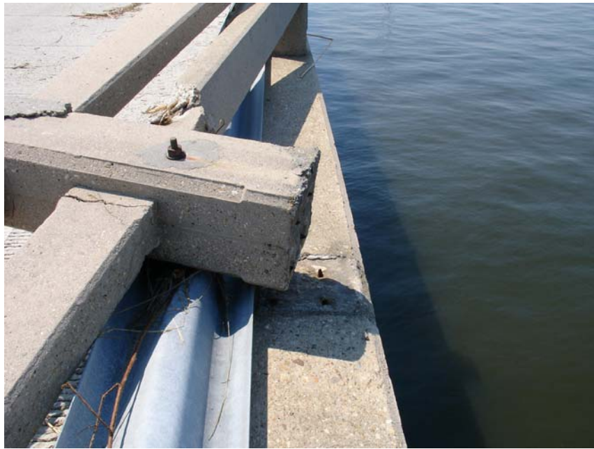
Figure 4 – Existing U.S. 11 Lake Pontchartrain Bridge Rail Damage
