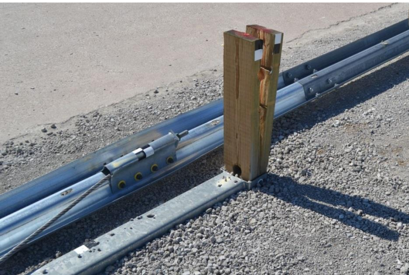
Figure 28. Upstream Anchor Damage, Test No. MGSMP-1
