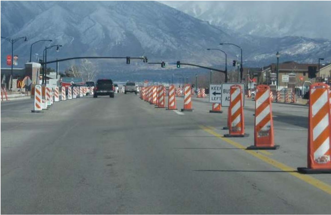
Figure 1. Improper sign height among channelizing devices.
