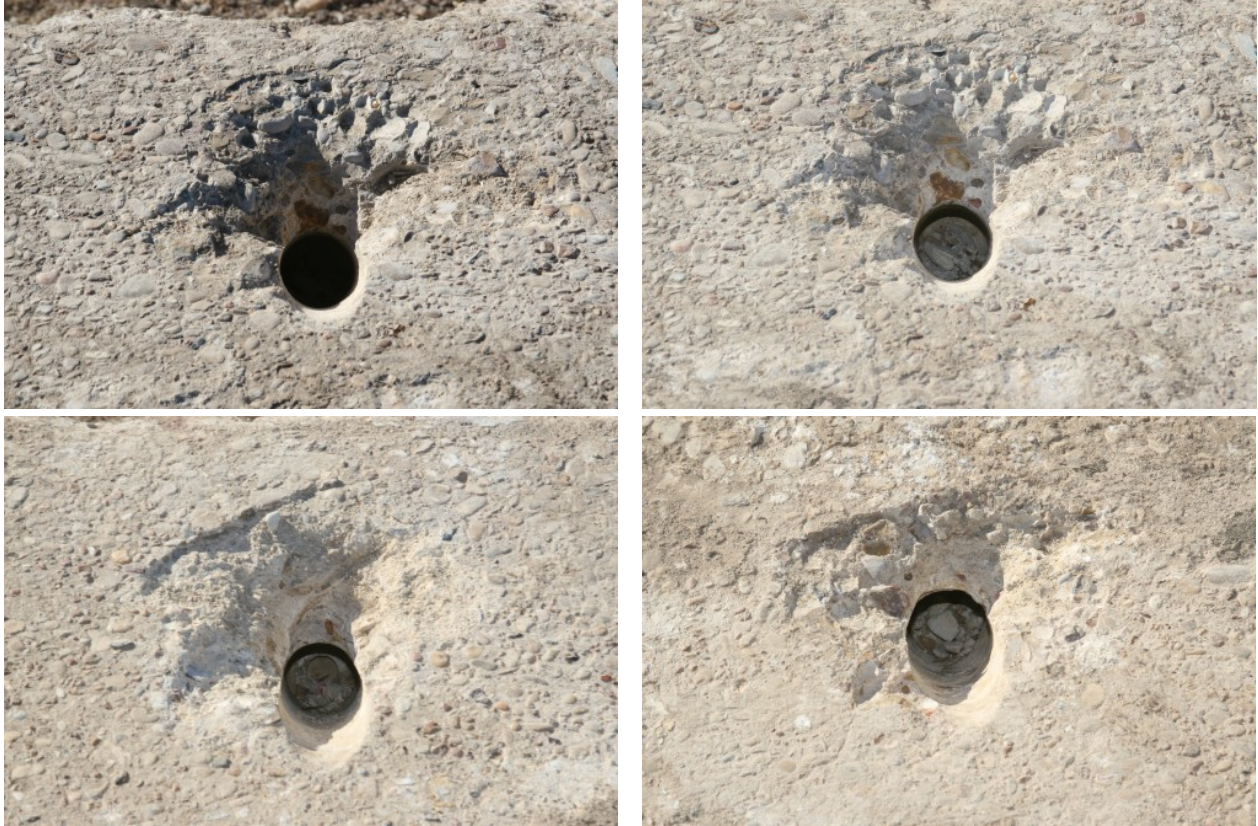
Figure 14. Holes in the underlying concrete pavement after the test.
