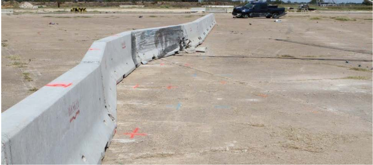
(Installation After Test)
