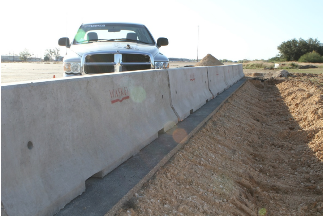
Figure 16. Test installation before test.
