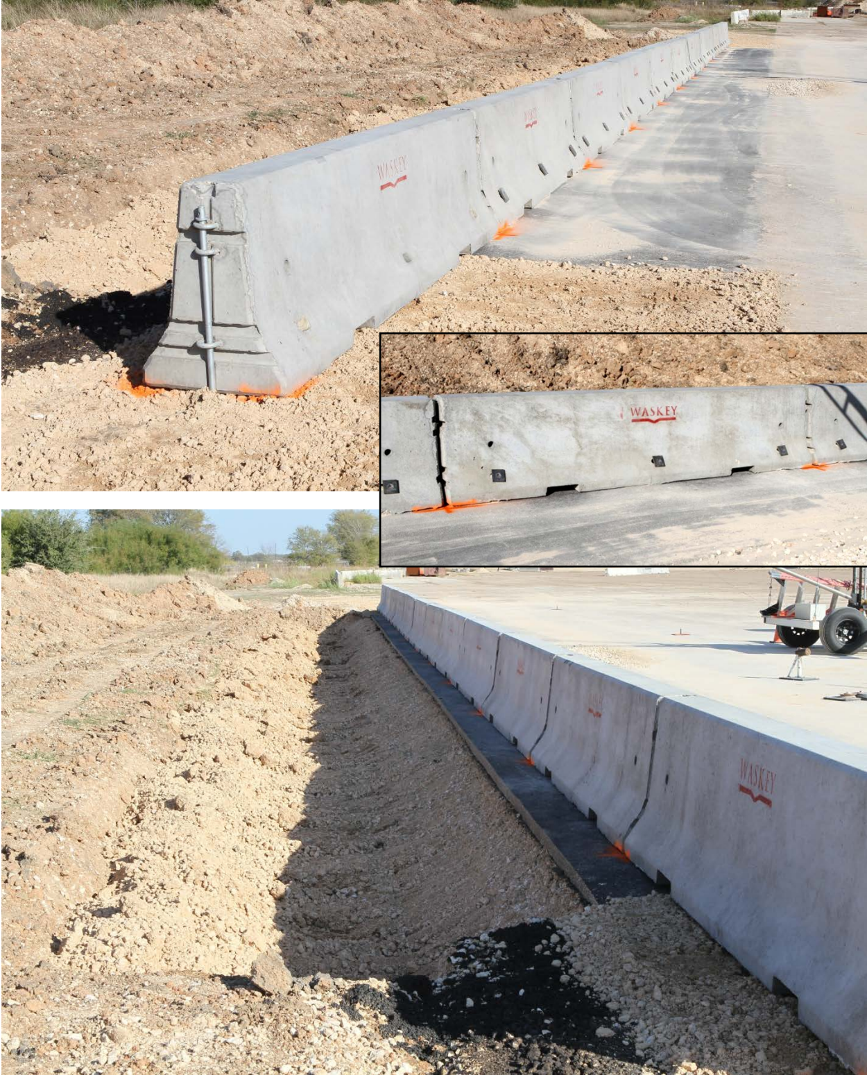
Figure 15. Pinned barrier installation on 4-inch asphalt past adjacent to a roadside slope.
