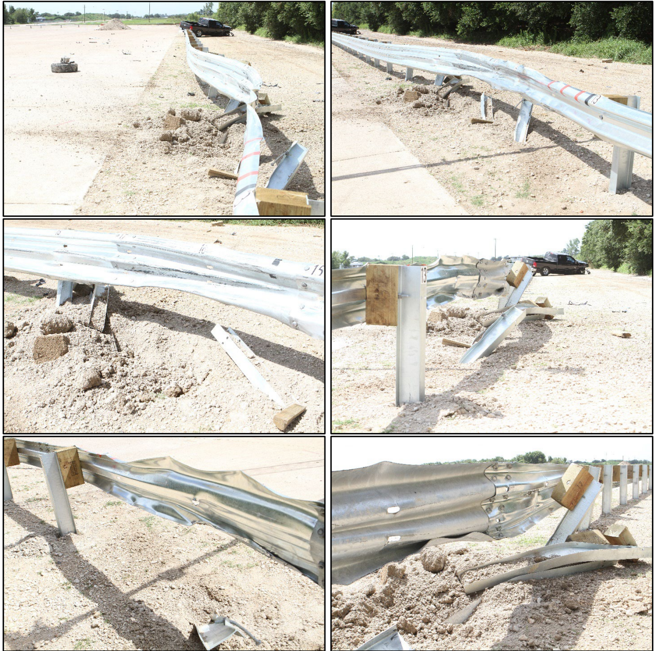
Figure 6.11. Roadside Thrie-beam after Test No. 614341-01-3.
