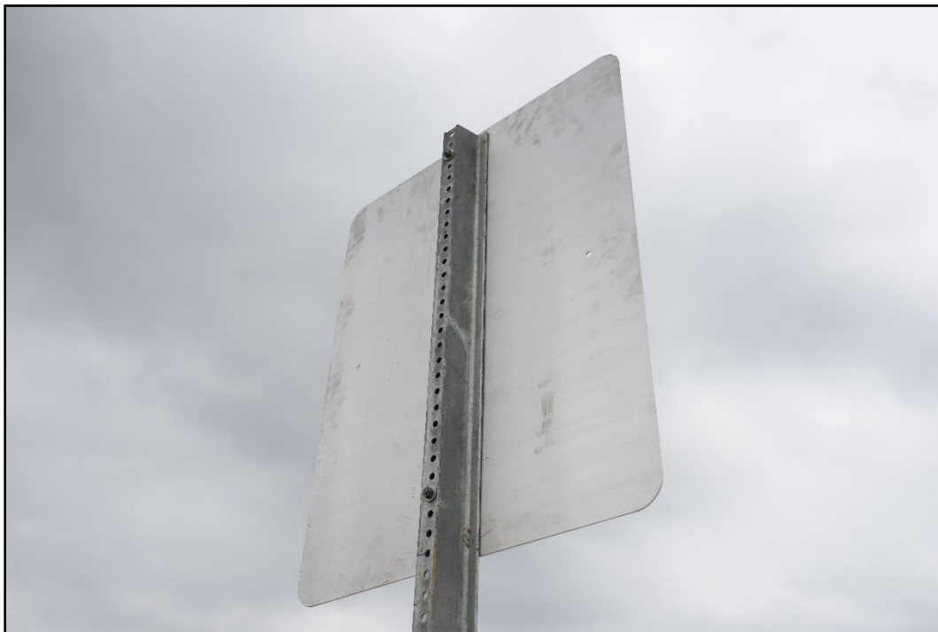
Figure 2.5. Rear Upper Section of the U-Channel Sign Support System prior to Testing.
