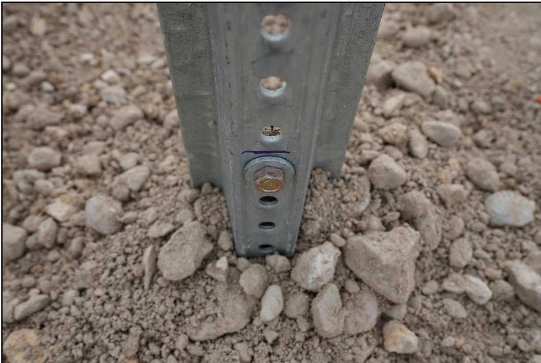
Figure 2.7. Ground Stub and Connection of the U-Channel Sign Support System prior to Testing.
