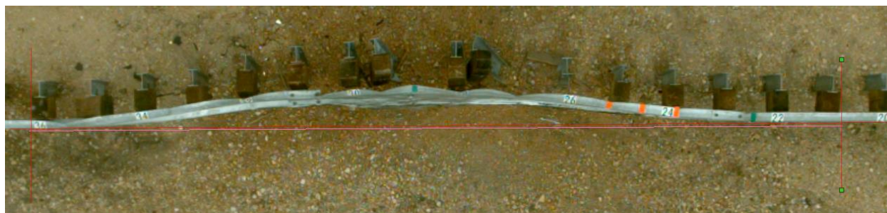
Figure 8.1. Width of Noticeable Damaged Section of Quarter Post Spacing System
