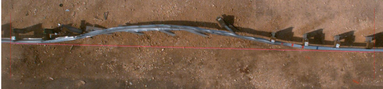
Figure 8.2. Width of Noticeable Damaged Section of Half Post Spacing System
