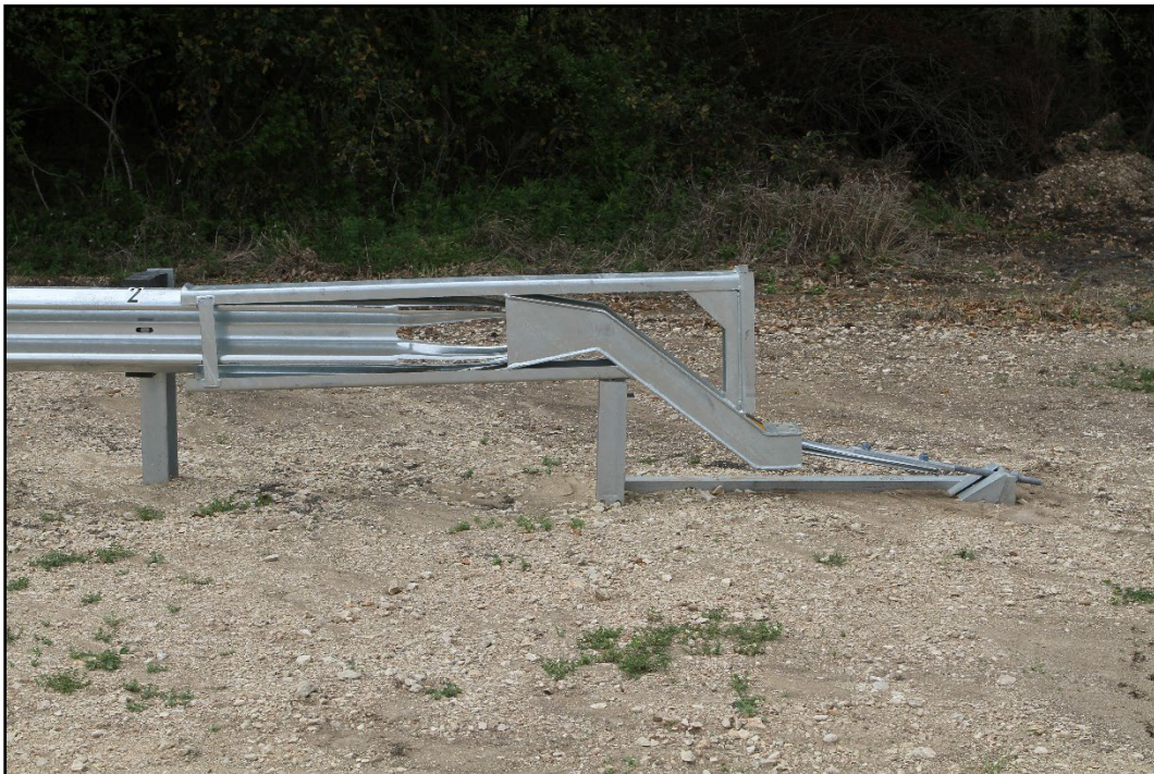
Figure 2.13. Upstream Terminal of the MGS Guardrail with Shortened 11:1 Flare prior to Testing.
