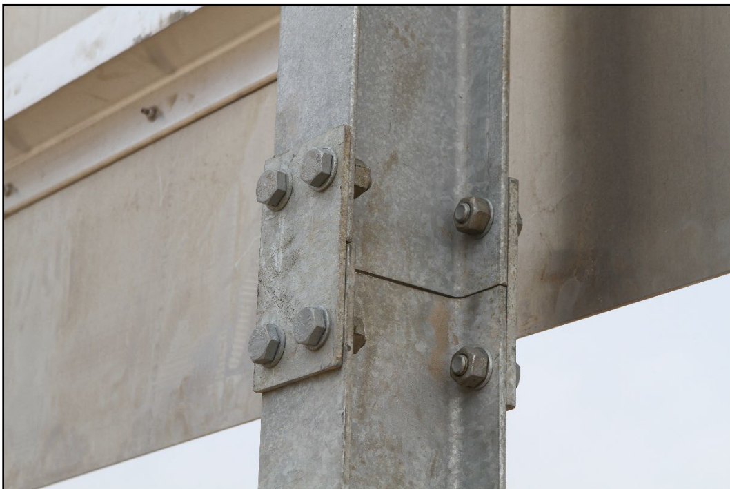
Figure 2.5. Hinge Plate of the Large Sign Slip Base Support Prior to Testing 612261-05-1.
