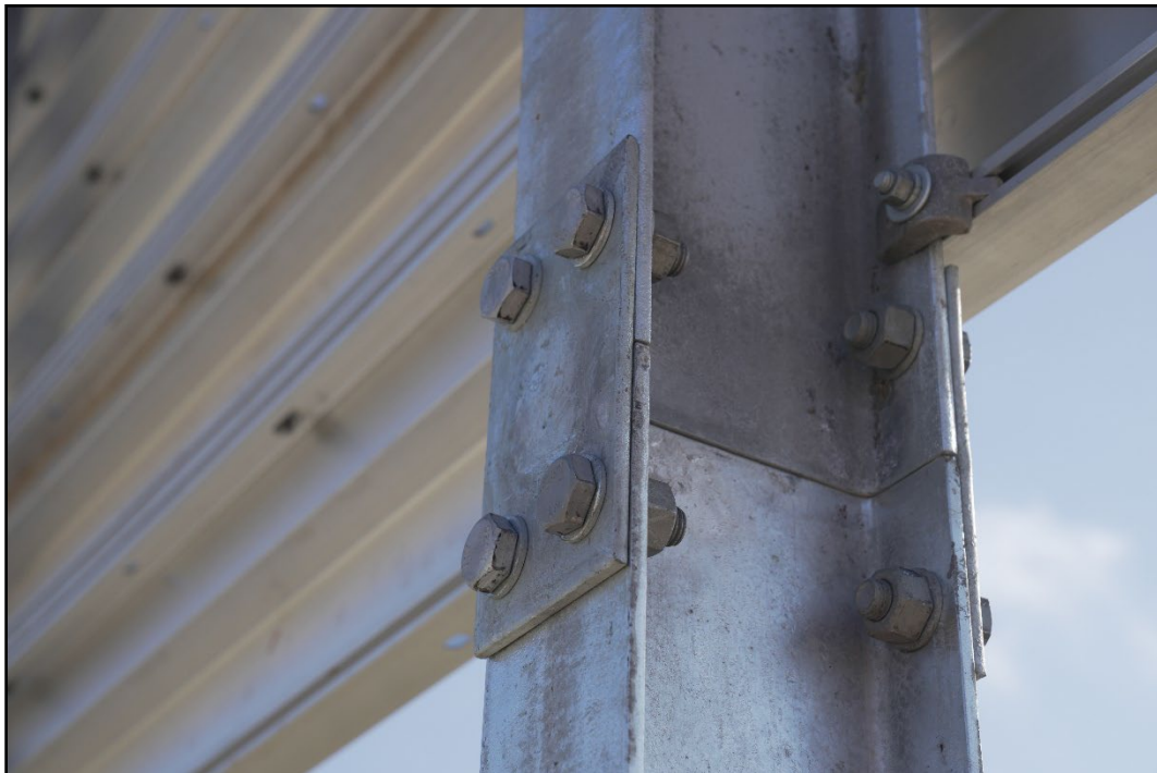
Figure 2.19. Hinge Plate of the Large Sign Slip Base Support on a Slope Prior to Testing 612261-05-2.
