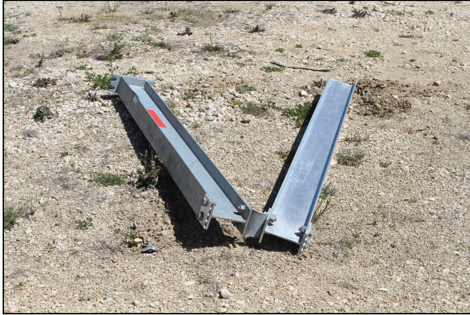
Figure 6.6. Impacted Post of the Large Sign Slip Base Support after Test 612261-04-1.
