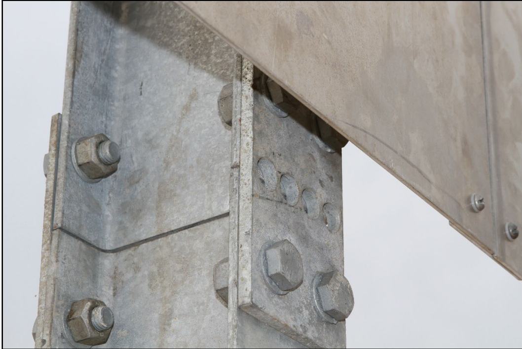
Figure 2.4. Front Plate of the Large Sign Slip Base Support Prior to Testing 612261-05-1.
