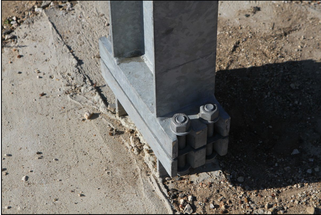
Figure 2.13. Impact Side of the Base of the Large Sign Slip Base Support Prior to Testing 612261-04-1.
