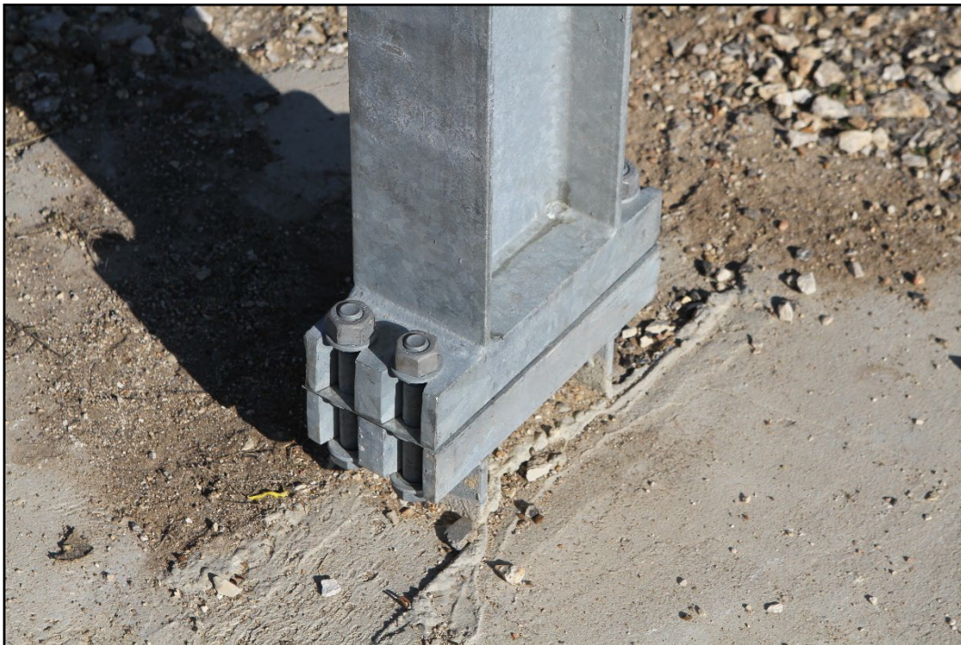
Figure 2.14. Opposite of the Impact Side of the Base of the Large Sign Slip Base Support Prior to Testing 612261-04-1.
