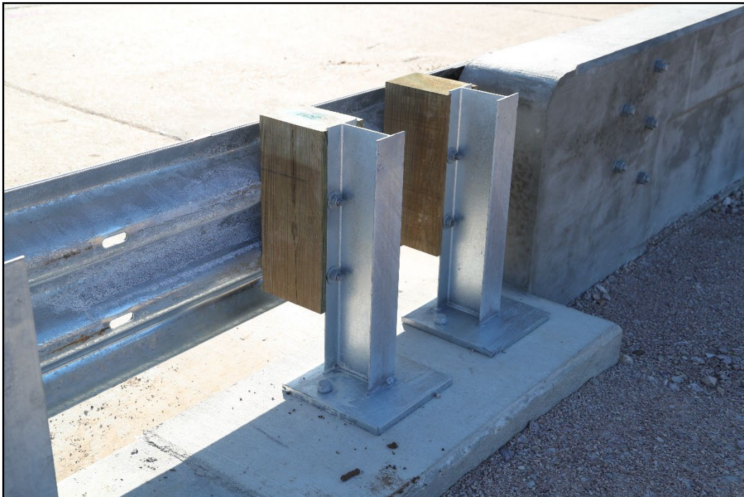
Figure 5.7. Field Side view of the Transition with Storm Drain Inlet Prior to Testing.
