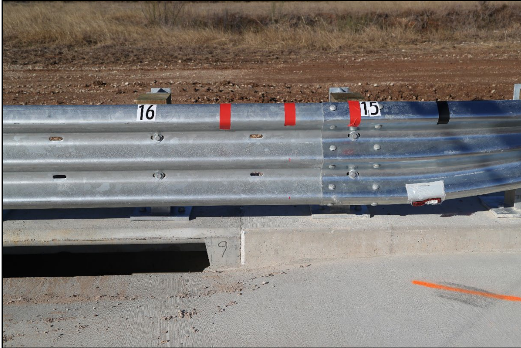
Figure 5.4. Transition with Storm Drain Inlet at Impact Prior to Testing.
