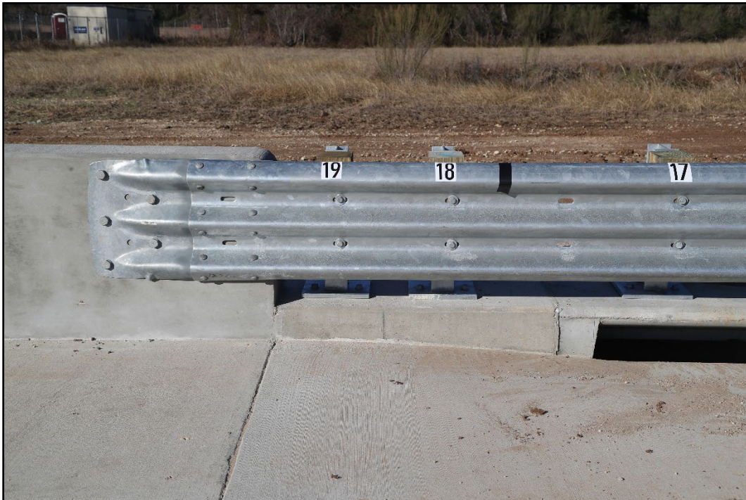
Figure 5.5. Thrie Beam to Parapet Connection for the Transition with Storm Drain Inlet Prior to Testing.
