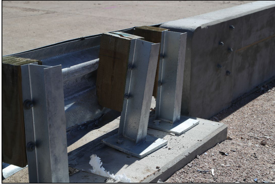
Figure 8.6. Field Side of the Transition with Storm Drain Inlet after Test 615251-01-1.
