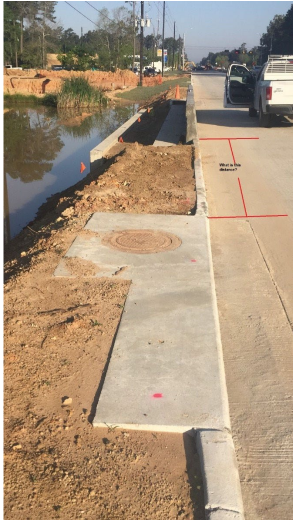
Figure 1. Example of a Storm Inlet.
