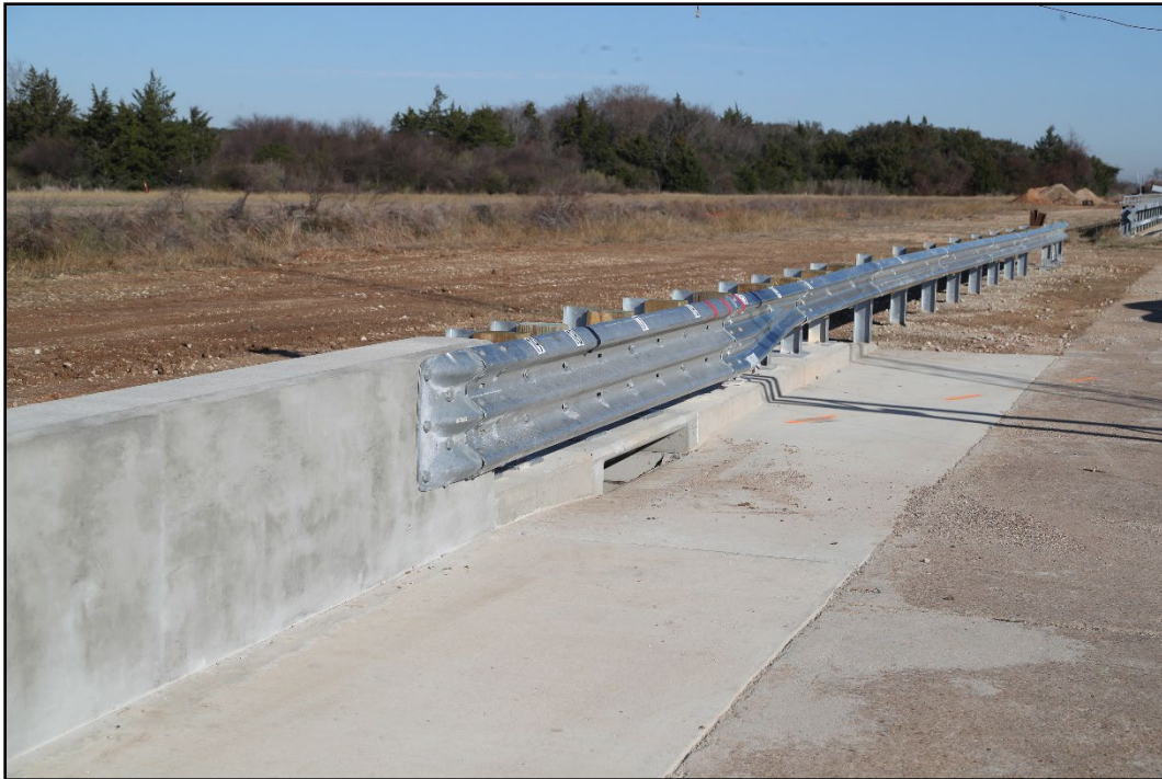
Figure 5.2. Downstream View of the Transition with Storm Drain Inlet Prior to Testing.
