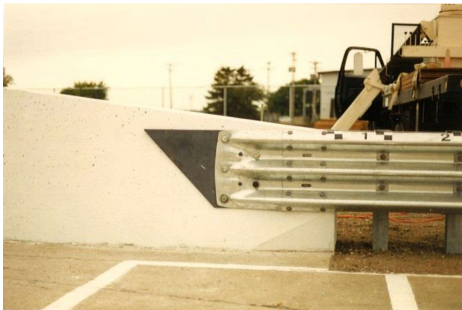
Figure 2.3. Single-Slope Concrete Median Barrier with 8:1 Height Transition for Attachment to Thrie-Beam Transition [9].
