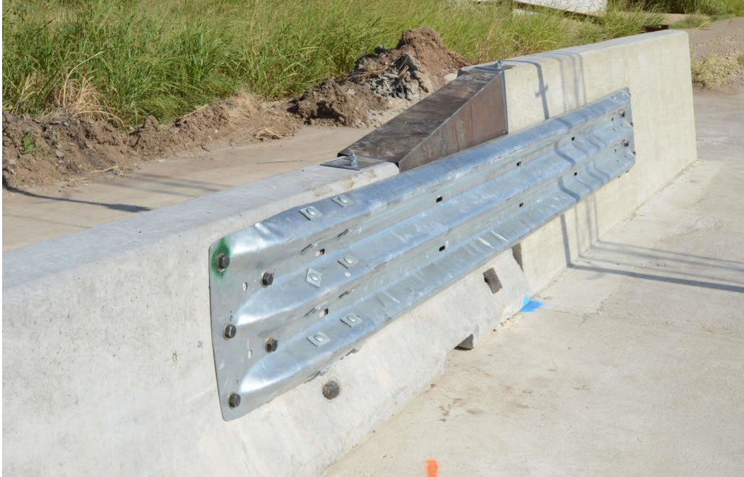
Figure 2.5. Transition Design for Anchored F-shape PCB to Rigid Vertical Concrete Barrier (Traffic Side) [11].
