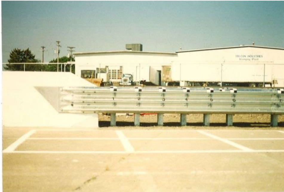
Figure 2.2. Single-Slope Concrete Median Barrier with 2:1 Height Transition for Attachment to Thrie-Beam Transition [8].
