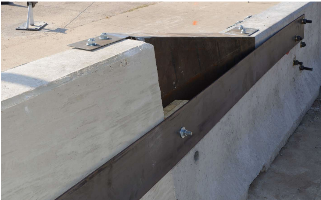
Figure 2.6. Transition Design for Anchored F-shape PCB to Rigid Vertical Concrete Barrier (Field Side) [11].
