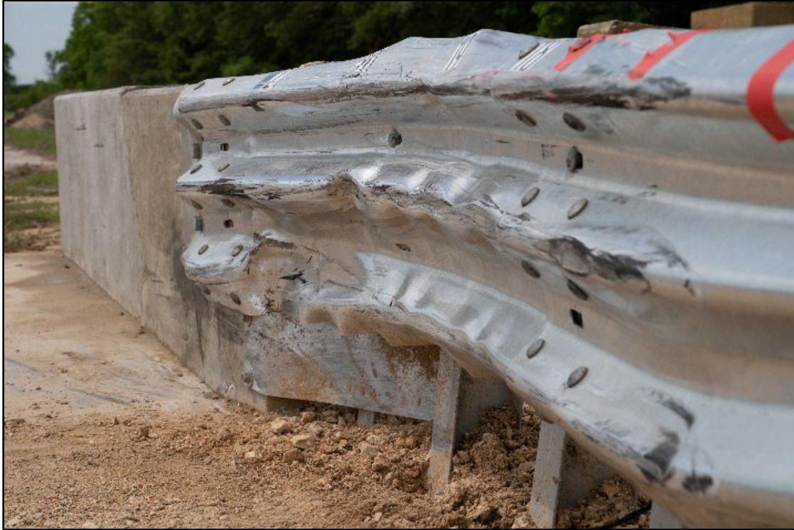
Figure 2.12. Damage Resulting from Snagging Interaction of Pickup Truck [15].
