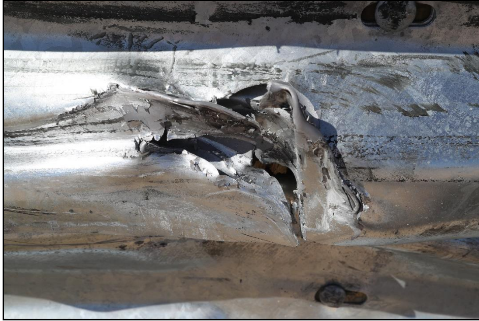
Figure 6.6. Vehicle Snag at Post 18 on the Median Guardrail Transition to Median F-Shape Barrier after Test 618851-01-1.
