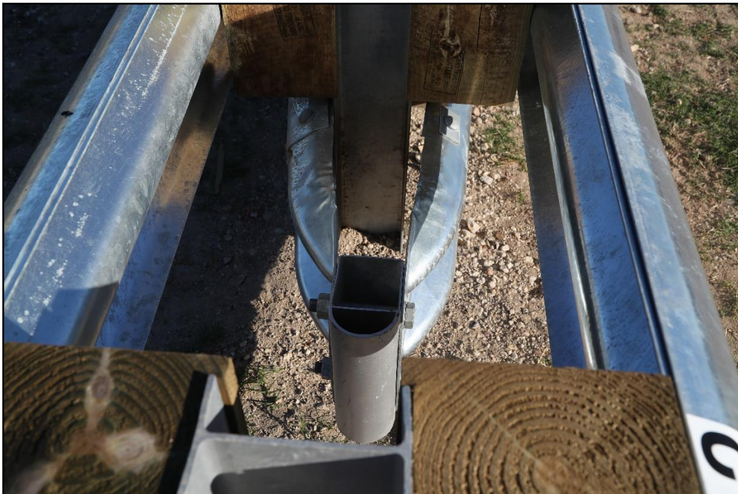
Figure 3.5. Median Guardrail Transition to Median F-Shape Barrier Upstream Rub Rail Termination prior to Testing.
