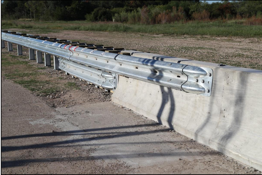
Figure 3.6. Downstream View of the Median Guardrail Transition to Median F-Shape Barrier prior to Testing.
