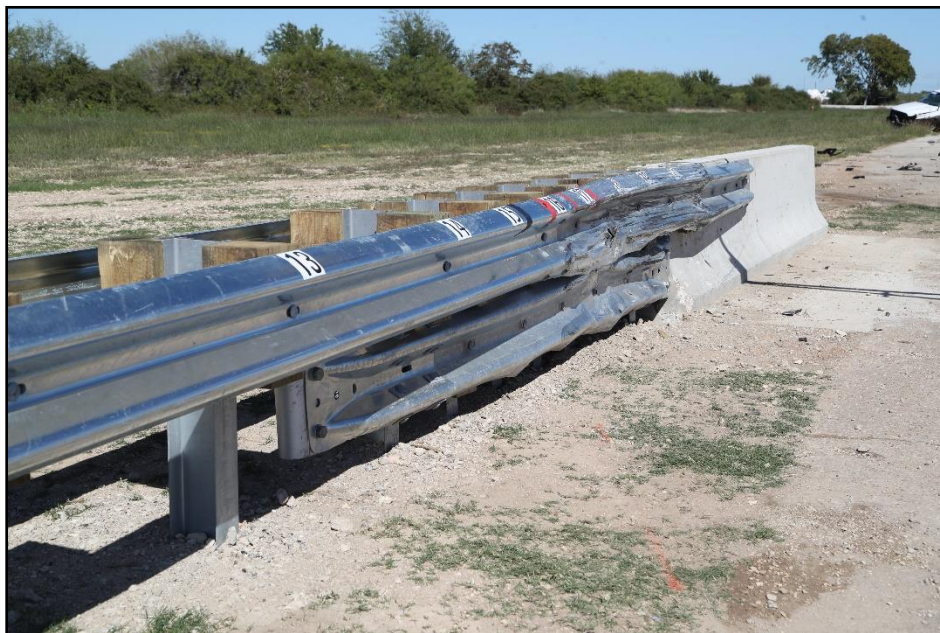
Figure 6.5. Median Guardrail Transition to Median F-Shape Barrier at Impact Location after Test 618851-01-1.
