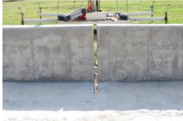
Figure 1.1. Example of Joint Opening in Concrete Bridge Rail (5).
