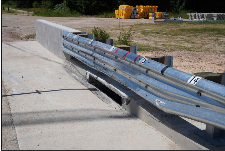
Figure 5.5. Traffic Side of the TL-3 Transition with a Storm Drain Inlet at Impact Location after Test 619551-01-1.
