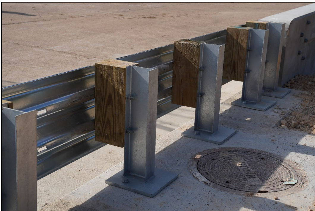
Figure 2.5. Field Side View of the TL-3 Transition with a Storm Drain Inlet prior to Testing.
