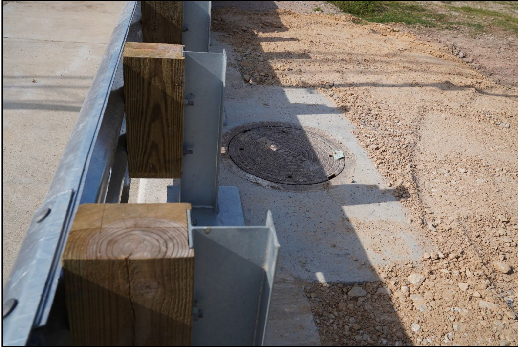
Figure 2.4. In-line View of the TL-3 Transition with a Storm Drain Inlet prior to Testing.
