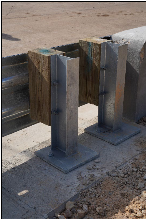
Figure 2.7. Posts of the TL-3 Transition with a Storm Drain Inlet at the Transition prior to Testing.
