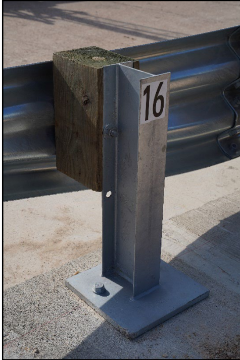
Figure 2.6. Post 16 of the TL-3 Transition with a Storm Drain Inlet prior to Testing.
