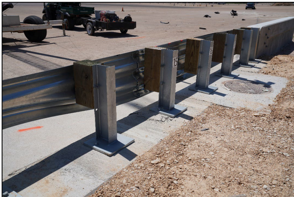
Figure 5.6. Field Side of the TL-3 Transition with a Storm Drain Inlet at Impact Location after Test 619551-01-1.
