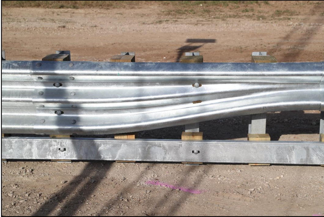
Figure 3.6. Traffic Side View of Shortened Transition at Thrie-beam Asymmetric Transition prior to Testing.
