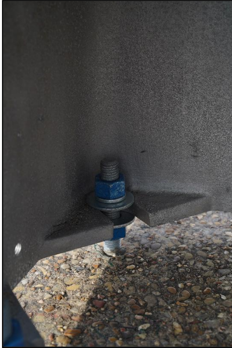
Figure 4.20. MUTCD Standard Pedestrian Signal Anchor Bolts Prior to Crash Tests 617891-01 3&4.
