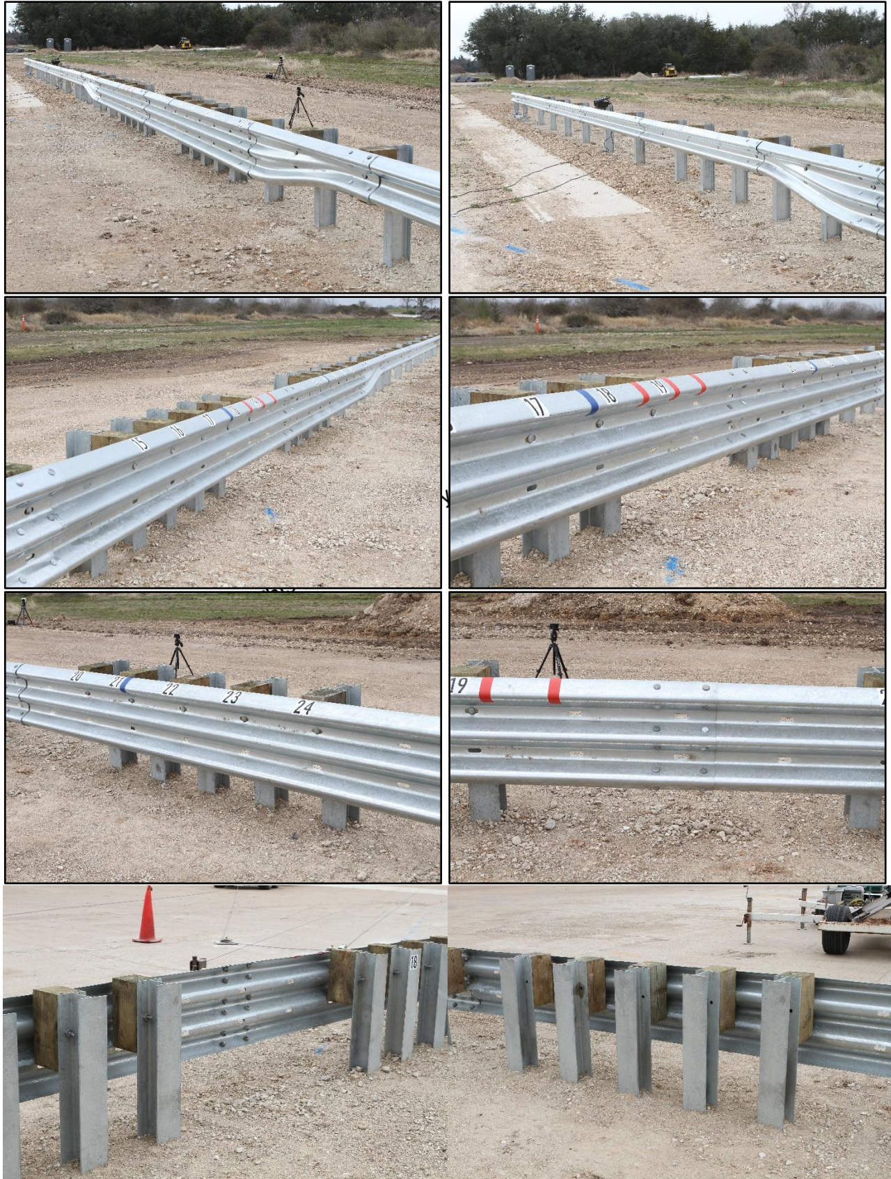
Figure 3.2 Thrie-Beam Guardrail System at a Fixed Object prior to Testing.
