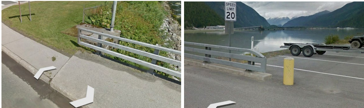
(a) “Do Nothing” approach at short radius turn (b) Bollard end; low-speed parking lot application
