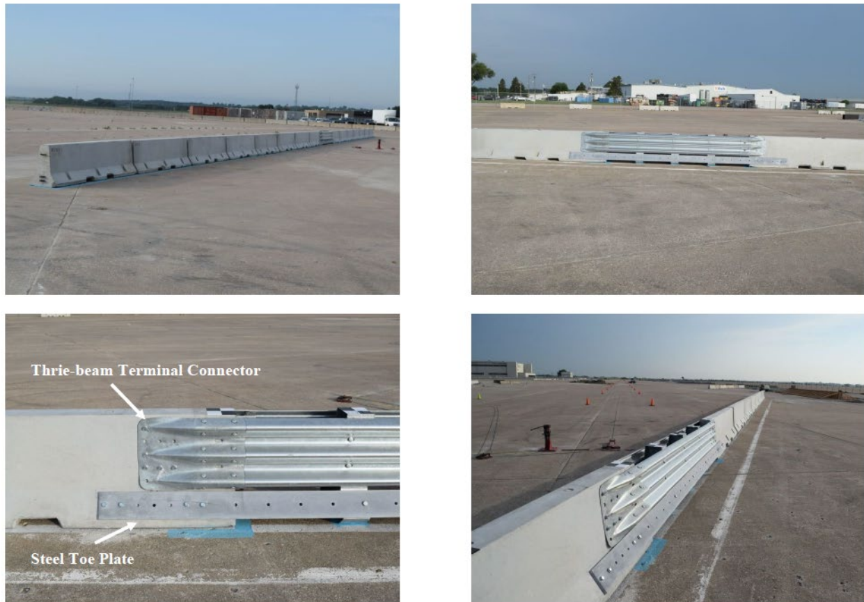
Figure 2.3. Bridging Large Opening Joints Between PCBs using Thrie-Beams and Steel Toe Plates [5, 6]
