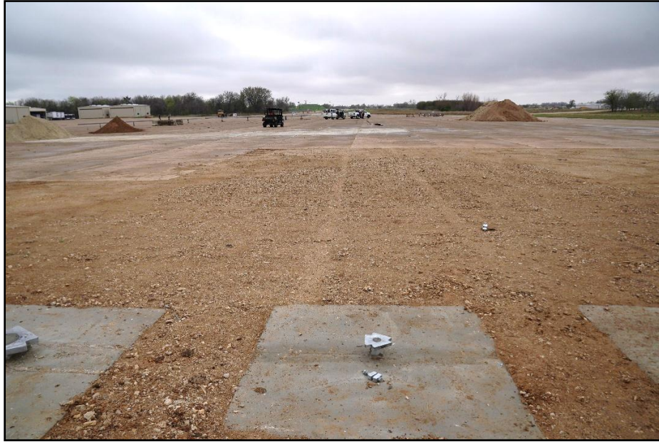
Figure 7.6. 3 × 3 Square Tube Slip Base Sign Support System at Impact Location after Test 621201-01-2.
